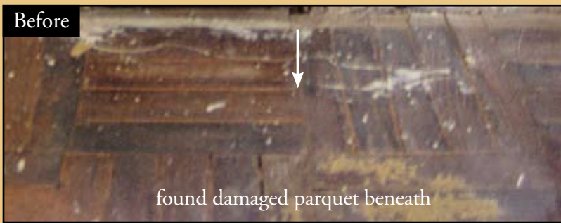
Wood parquet was stained and water damaged
